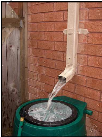
Figure. 4 Rainwater collection (through downpipes and sieves)
